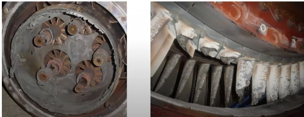
Fig: Damaged combustor [1].
